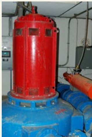
Buffalo Hydropower Plant
